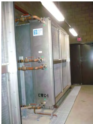
Cooling Water System
