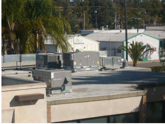
Rooftop HVAC Units
