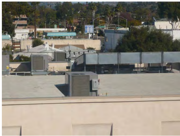
Rooftop Mechanical Equipment
