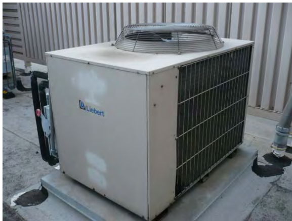
Rooftop Air Conditioner
