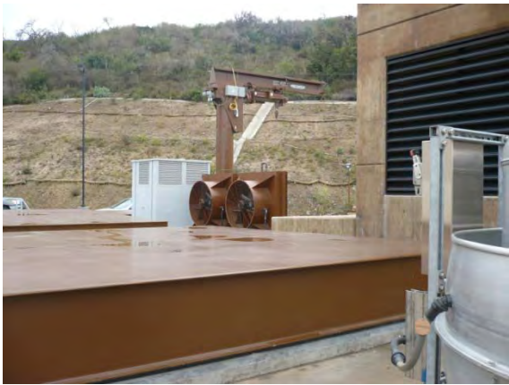
Top Hatch of Pump/Generator Station
