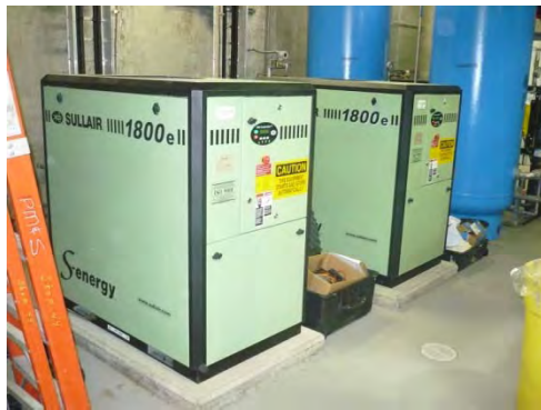
Support Equipment - Compressed Air System
