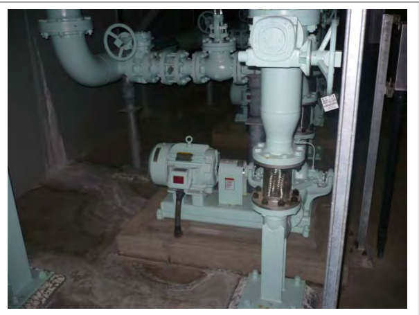
Service Water Pump
