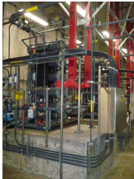
Sodium Hypochlorite Generation System
