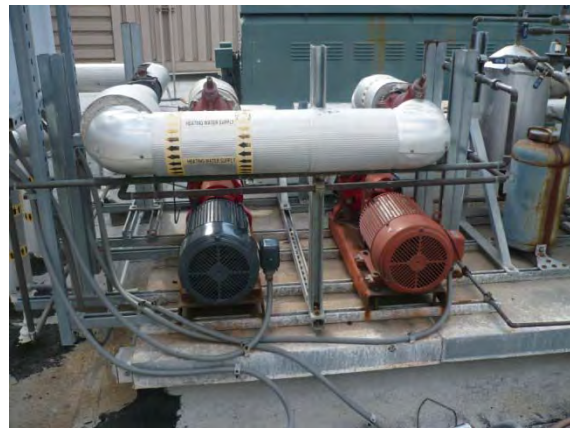
Hot Water Recirculation Pumps
