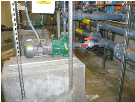
Chemical Water Mixing Pumps
