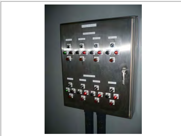
Service/Cooling Water Panel
